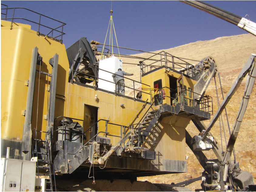
A crane lowers a new digital control system into an electric shovel.
