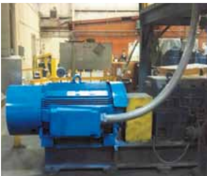
400 HP DC to AC Extruder Motor Conversion
