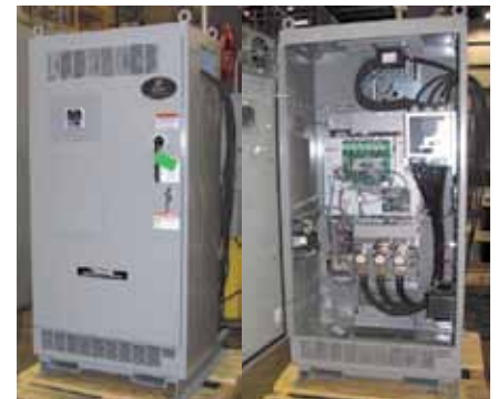
400 HP DC to AC Extruder Drive Conversion
