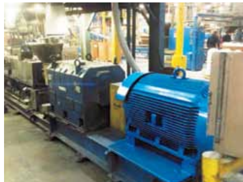
Extruder 2 - 400HP AC Motor as Installed
