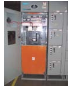
Inside Cabinet View with Door Open
